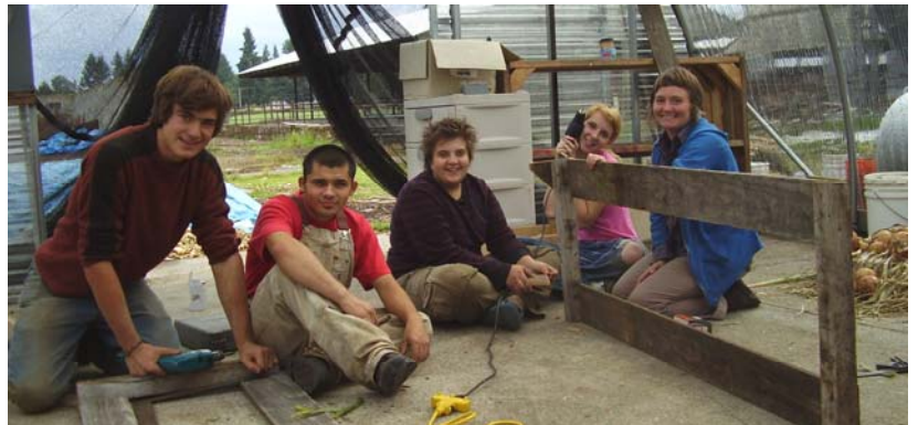
Youth and volunteers built a new chicken tractor at the volunteer day last Saturday. Thanks to volunteer Kellie Henwood, far right, for getting a donation of lumber for this project (from Olympia Salvage—Thank you!)
